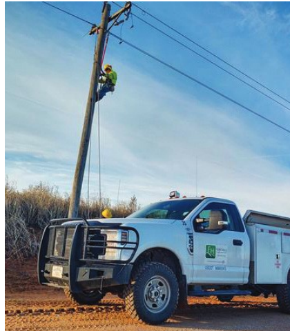
Flint Hills REC also sent a foreman's pickup truck, digger derrick, pole trailer, large bucket truck, and enough materials to frame 100 poles.
