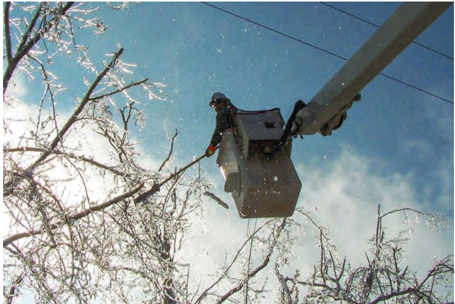
Clear power lines make it easier and safer for lineworkers to access lines and fix problems that occur.
